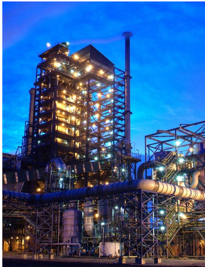
Figure 3: ISASMELT™ Plant at Mufulira Smelter.
