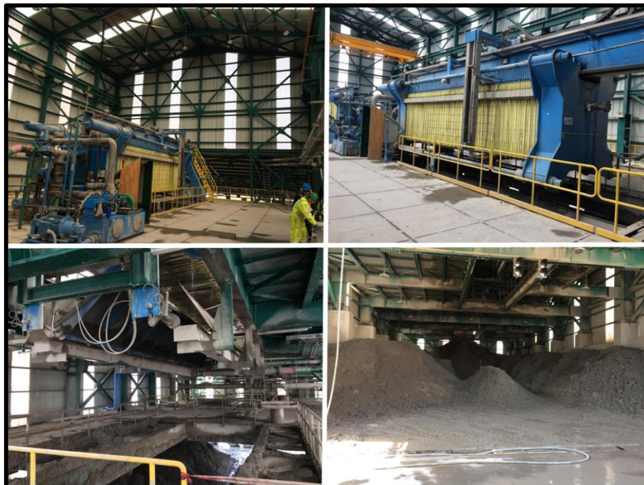
Figure 12: Multi-story filter press building at Buenaventura's Tambomayo mine.
