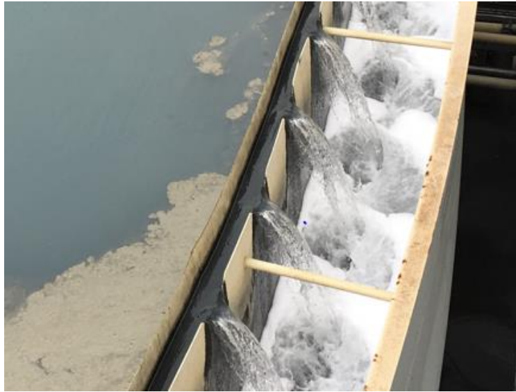
Figure 13: Typical overflow clarity on Thickener No. 1.
