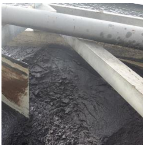
Figure 2: Sanding-out in channel.
