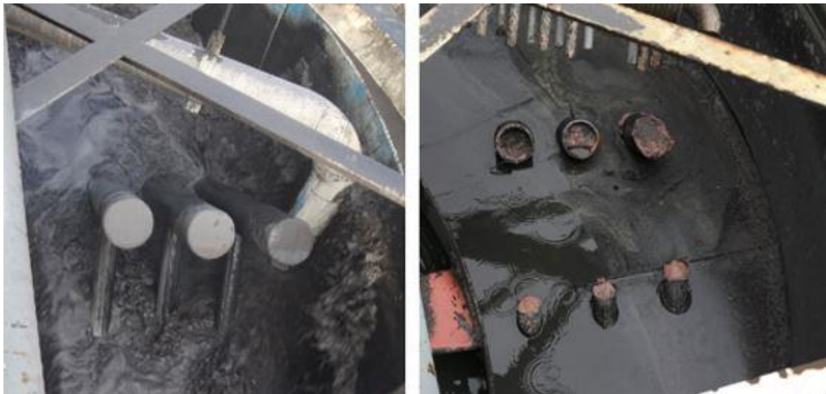
Figure 5: Mixing baffles and their removal.
