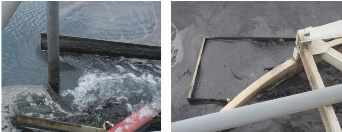
Figure 1: Feedwell dilution channels operating well and poorly.
