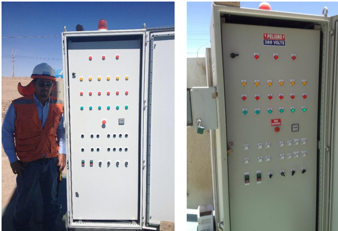
Figure 4. KIMBO control cabinet (HMI).
