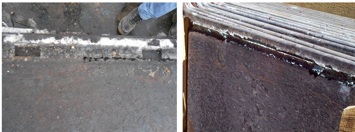
Figure 8. Corrosion at solution line by organics.
