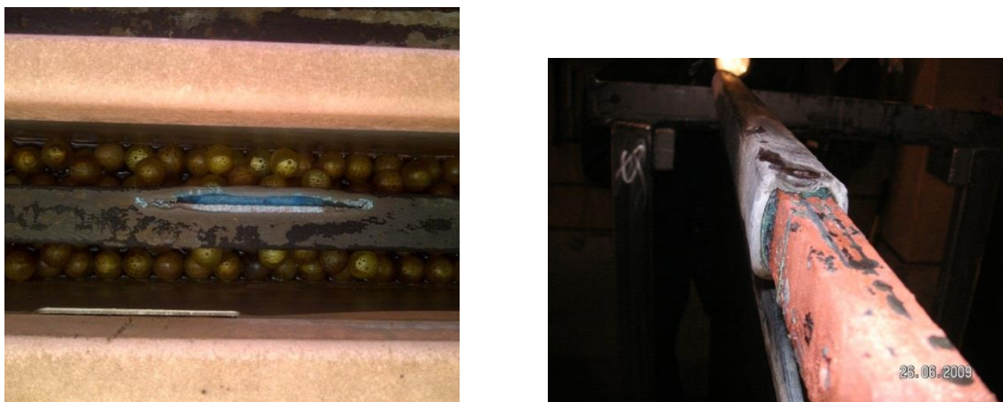
Figure 6. Corrosion of hanger bar by acid penetration.
