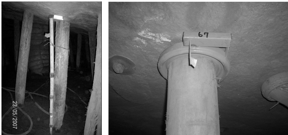
Figure 10. Closure and Load Loggers installed with a pencil prop in a platinum mine
