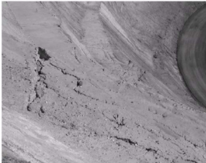
Figure 17 Cracking and slumping of a berm above the ramp.
