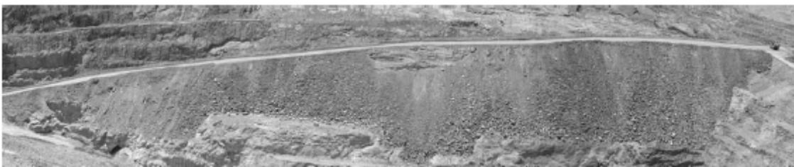
Figure 6 Rock fill buttress placed to increase stability of the main haulage ramp.
