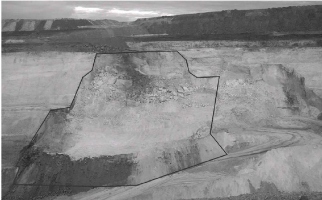
Figure 8 Harmony 1C Slip, showing existing failure to the right, with extension outlined.
