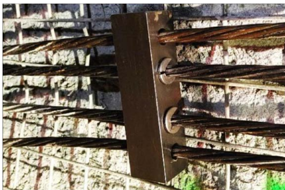
Figure 6—Connector block used to tension pillar wrap cable slings at the New Afton mine
