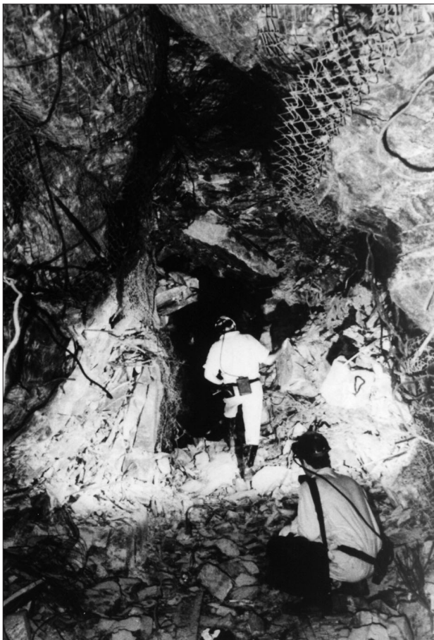
Figure 2—Adverse haulage conditions at Hartebeestfontein mine caused by large time dependent deformation and the eventual collapse of the support. Note that this is not rockburst damage (courtesy W.D. Ortlepp)
