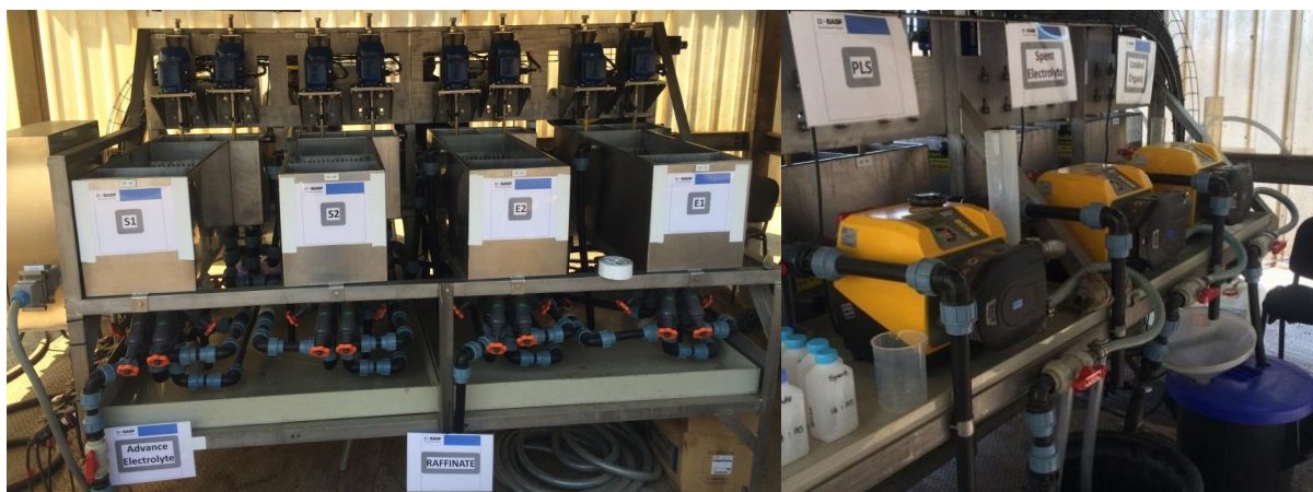
Figure 2. Pilot plant in operation at the commercial plant.
