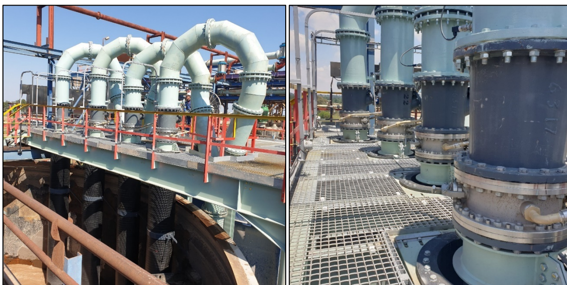
Figure 1. Site A: Plant Aachen installation pictures.
