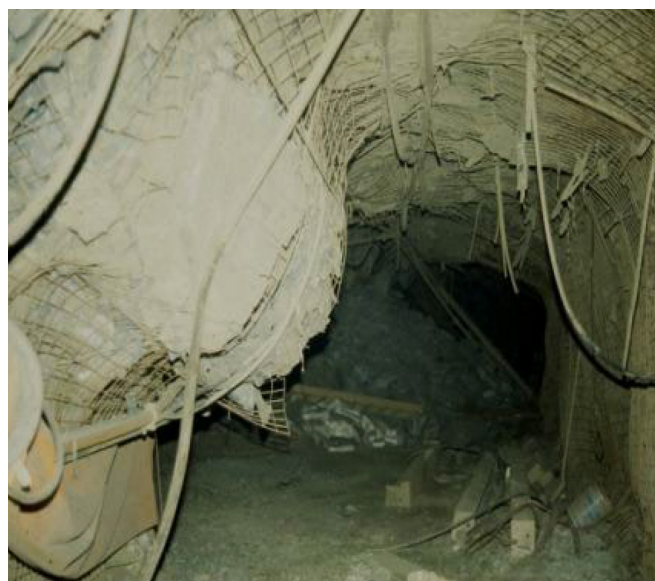
Figure 9—Support system damaged by a seismically triggered strainburst causing loading by rock mass bulking (Kaiser, Cai 2013)
