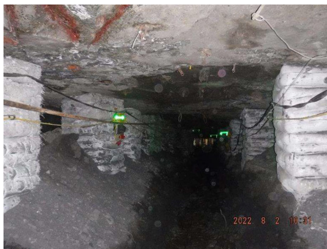
Figure 10—Winch PDS installation in raise line (Sibanye-Stillwater, 2024)
