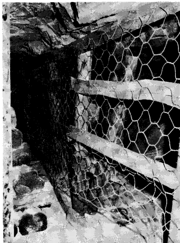
Fig. 6—Paddock construction showing the retaining mesh and split lagging supported on mine poles
