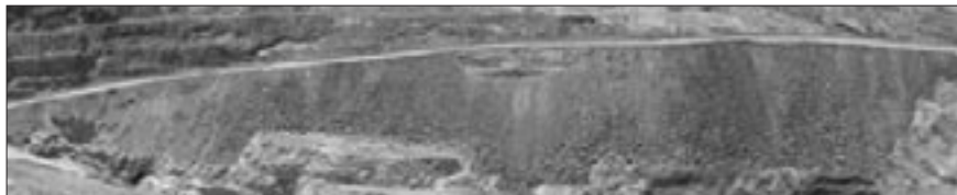
Figure 6—Rock fill buttress placed to increase stability of the main haulage ramp
