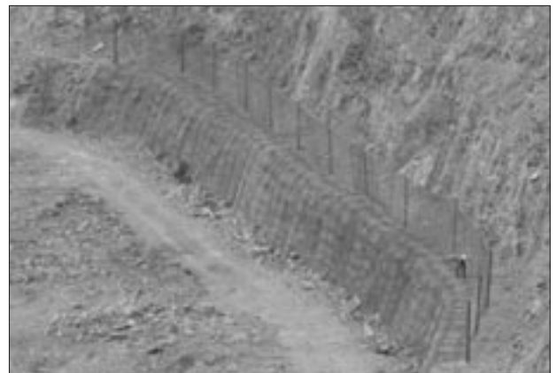
Figure 15—Catch fence and mesh curtain
