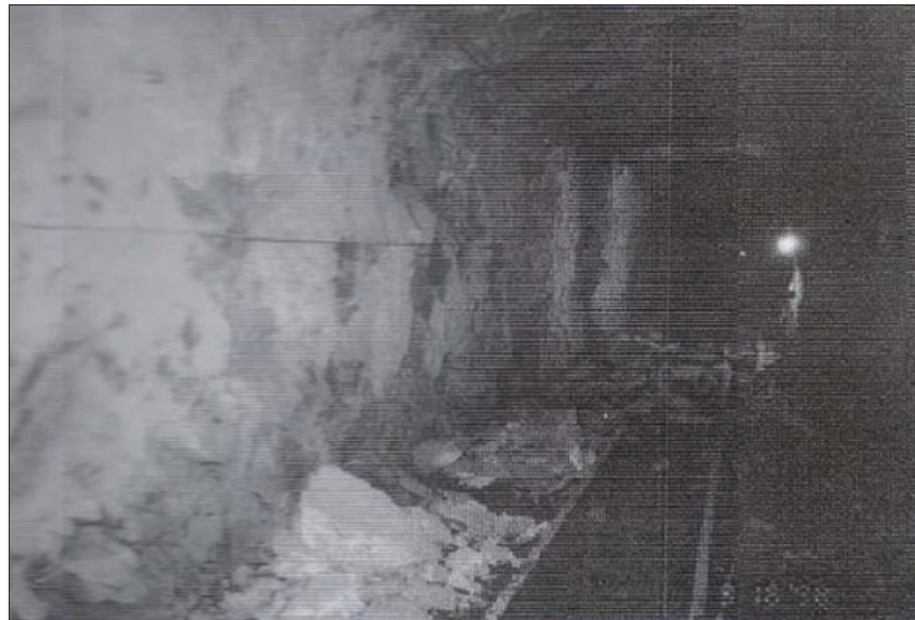
Figure 4—Photograph of ‘high intensity damage’ (sic) along experimental tunnel
