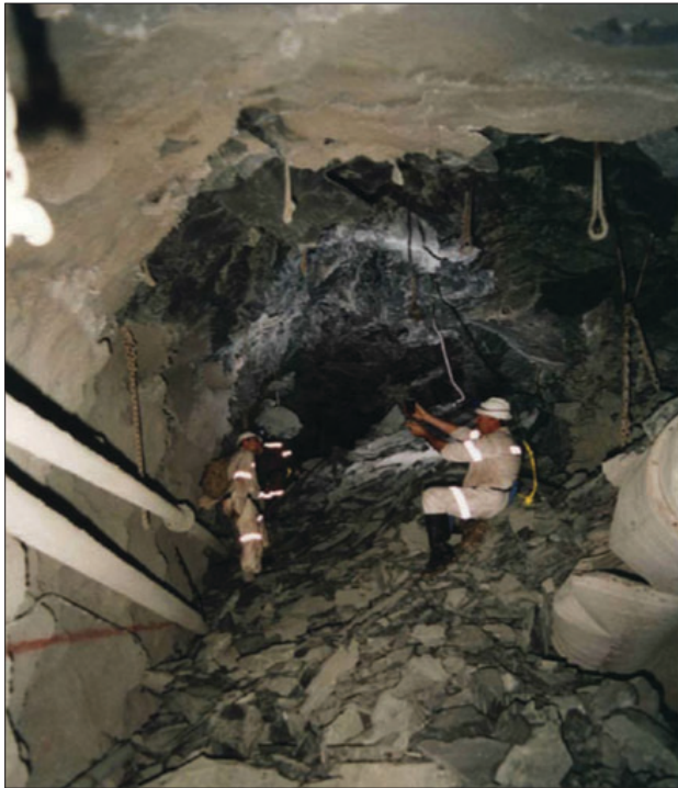
Figure 1—Severe rockburst damage in a deep tunnel approximately 60 m from its intersection with a fault on which a seismic event of M_L = 3,1 occurred
