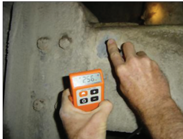
Figure 9—Examination of a shaft buntion. The underlying hot dip galvanized coating measured 256 \mu\text{m}
