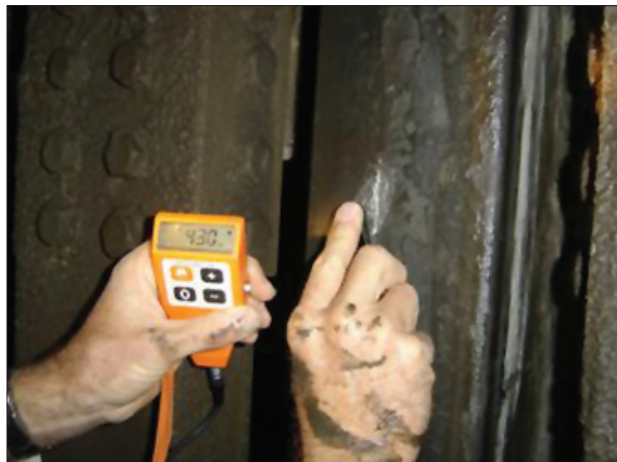
Figure 7—Examination of a shaft guide. Removal of the encrusted poultrices and measuring the underlying hot dip galvanized protective coating reveals a coating thickness of 430 \mu\text{m}
