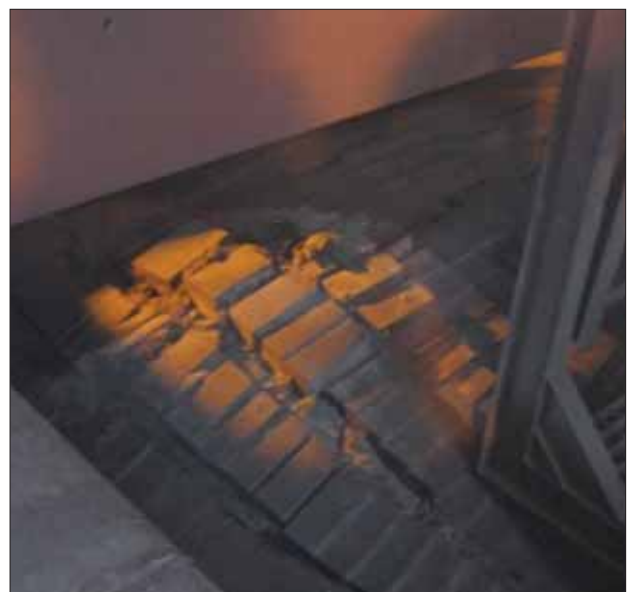
Figure 3—Reaction shaft roof damage
