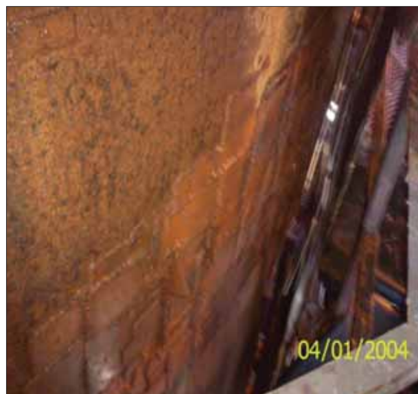
Figure 4—Typical patch ongoing repairs after six months of operation to reaction shaft shell
