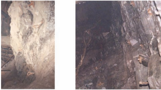
Figure 1—Structural failures in orepasses
