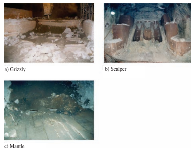
Figure 5—Block size control infrastructure: (a) grizzly, (b) scalper, and (c) mantle
