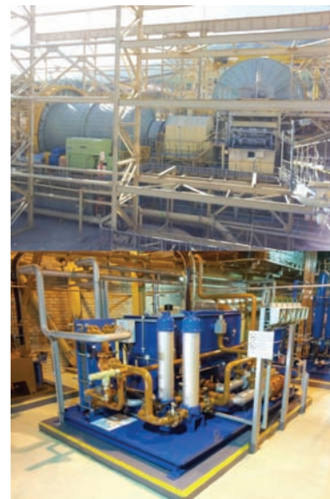
Figure 11—Mills and lube rooms
