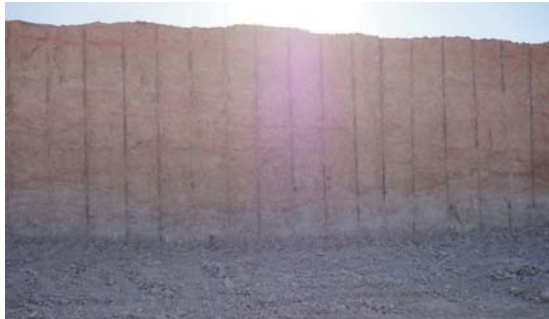
Figure 9—Example of good results achieved in calcrete
