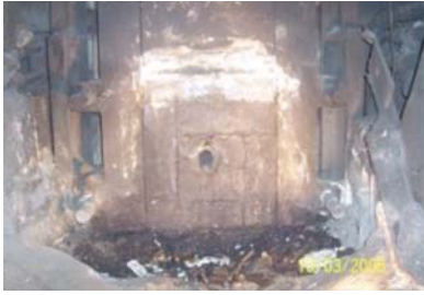
Figure 14—Water-cooled 'dogbox' with minor cracks in surround bricks around tapping module brick with '+-shaped' crack and off-centre drill-hole (Nelson et al. , 2007)
