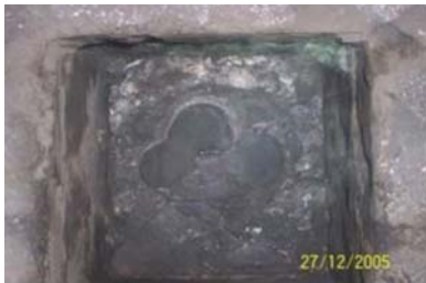
Figure 15—Tapping module brick 4 after 219 taps. Multiple drillings of the tap-hole are off-centre, and are coupled with skew lancing (Nelson et al. , 2007)
