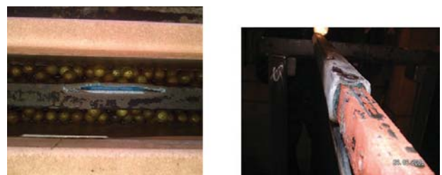
Figure 6—Corrosion of hanger bar by acid penetration
