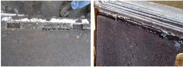
Figure 8—Corrosion at solution line by organics
