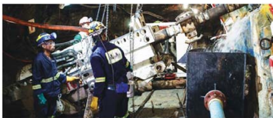
Figure 21—Reef boring rig, with water and chip capture on right (AngloGold Ashanti)
