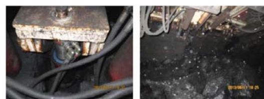
(a) support leakage
