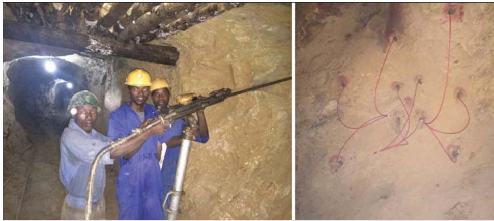
Figure 3—Underground rock-drilling and completed development round (11 holes) utilizing a 5-hole burn cut
