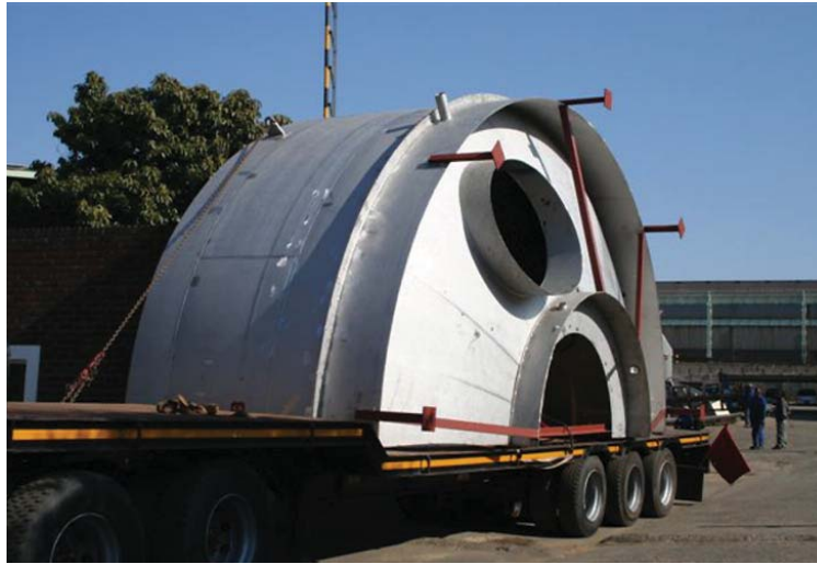
Figure 7—Prefabricated converter modules
