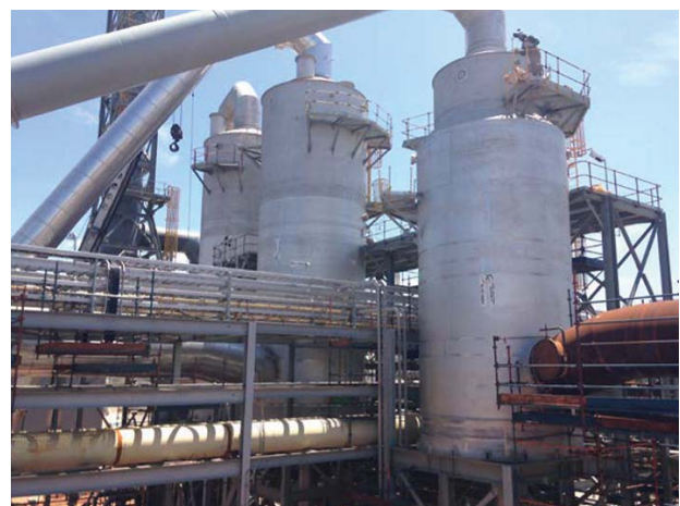
Figure 2—SARAMET™ acid towers in installed position
