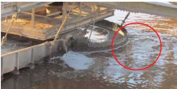
Figure 13—Problematic flow patterns resulting from thickener feedwell arrangement
