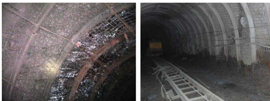
Figure 9—Coated drifts in Omerler underground coal mine
