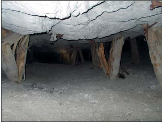
Figure 10—Photograph of the panel along the down-dip side of pillar 16. The elongates were damaged during the seismic event. There were also signs of footwall heave
