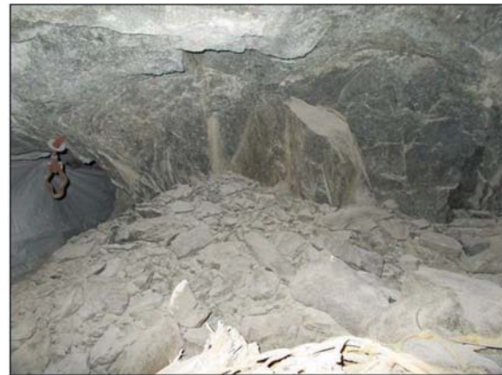
Figure 7—Condition of pillar 1. The pillar was situated adjacent to a pothole, which prevented the pillar from crushing
