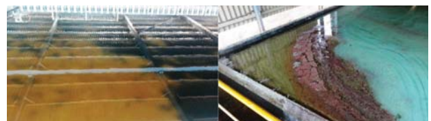
Figure 10—Crud formation in the diluent wash (left) and strip settler (right)
