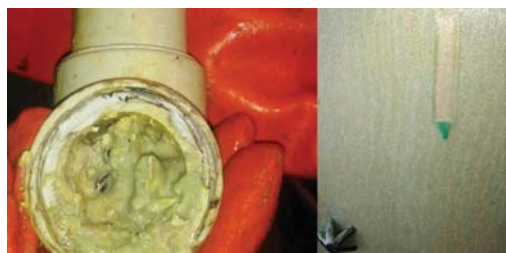
Figure 5—(Left) Pipe blockages from colloidal silica formation, (right) silica gel precipitation on tankhouse anodes
