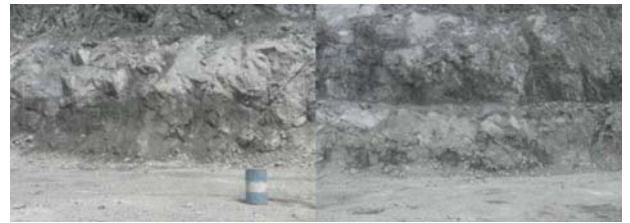
Figure 2—Western highwall showing crest damage and highwall damage
