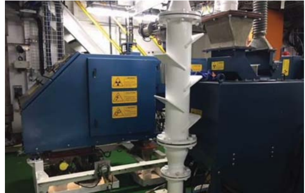
Figure 5—XRT reconcentration machine (BDT1122) installed on a Debmarine Namibia mining vessel. The machine processes the final recovery plant concentrate before canning
