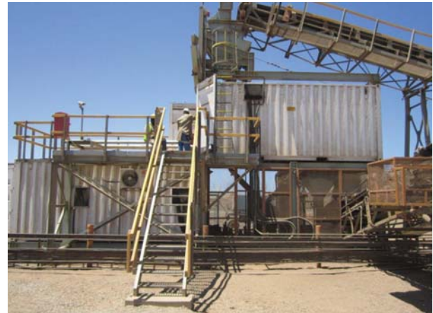
Figure 7 – The XRT pilot plant installation in Oranjemund, Namibia. The system consisted of a containerized high-throughput machine coupled with a container housing the services required to run the plant
