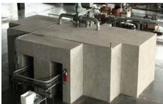
Figure 1—Protective bunker with a height of 2.3 m for the LINAC with an energy of 3 MeV
