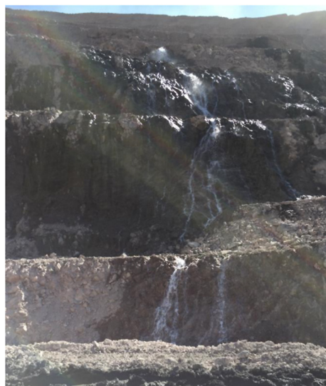
Figure 1—Water pouring from a pit slope, affecting stability and production
