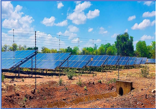
Figure 9—Photovoltaic solar panels (1,037 kWp) at TCM
