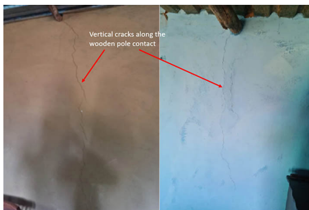
Figure 2—Vertical cracks at wood lintels running straight down to the floor
