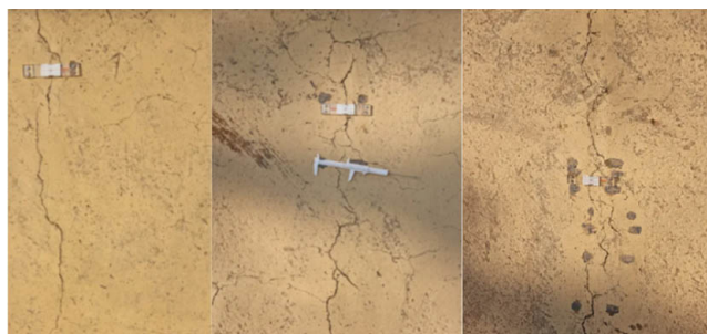
Figure 1—Vertical cracks with crack monitors installed
