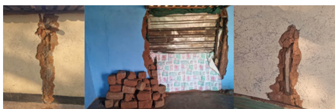
Figure 3—Vertical cracks between the vertical poles and major failure in between
