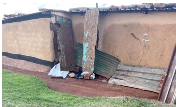
Figure 4—Moisture on the wall and heavy loose material on the roof introducing load and vibration
