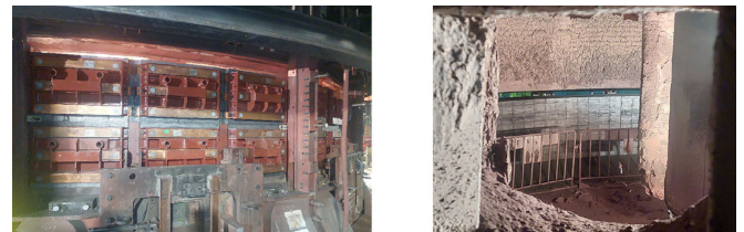
Figure 7—Reinstalled copper-graphite composite coolers from (a) the outside, and (b) from inside through the furnace freeboard inspection port
