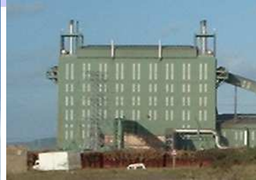
Furnace Gas Cleaning Plant during normal operation : -no visible flame -emissions far below legal requirements -safe furnace and gas plant operation -furnace pressure controlled CO gas extraction
