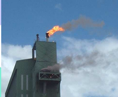
Furnace Gas Cleaning Plant venting during Emergency Situation, e.g.: -power failure -scrubber water failure -unacceptable O 2 concentration level
