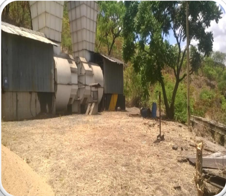
NEGATIVE PRESSURE AXIAL FANS AT TROJAN
