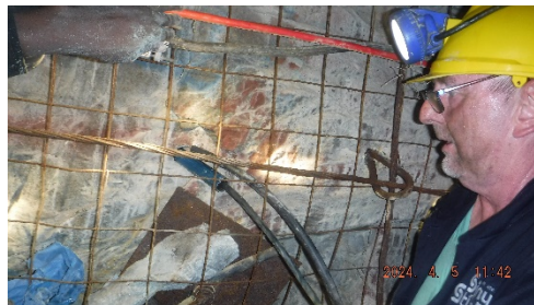
Figure 5. The installation of the 8 G accelerometer.
