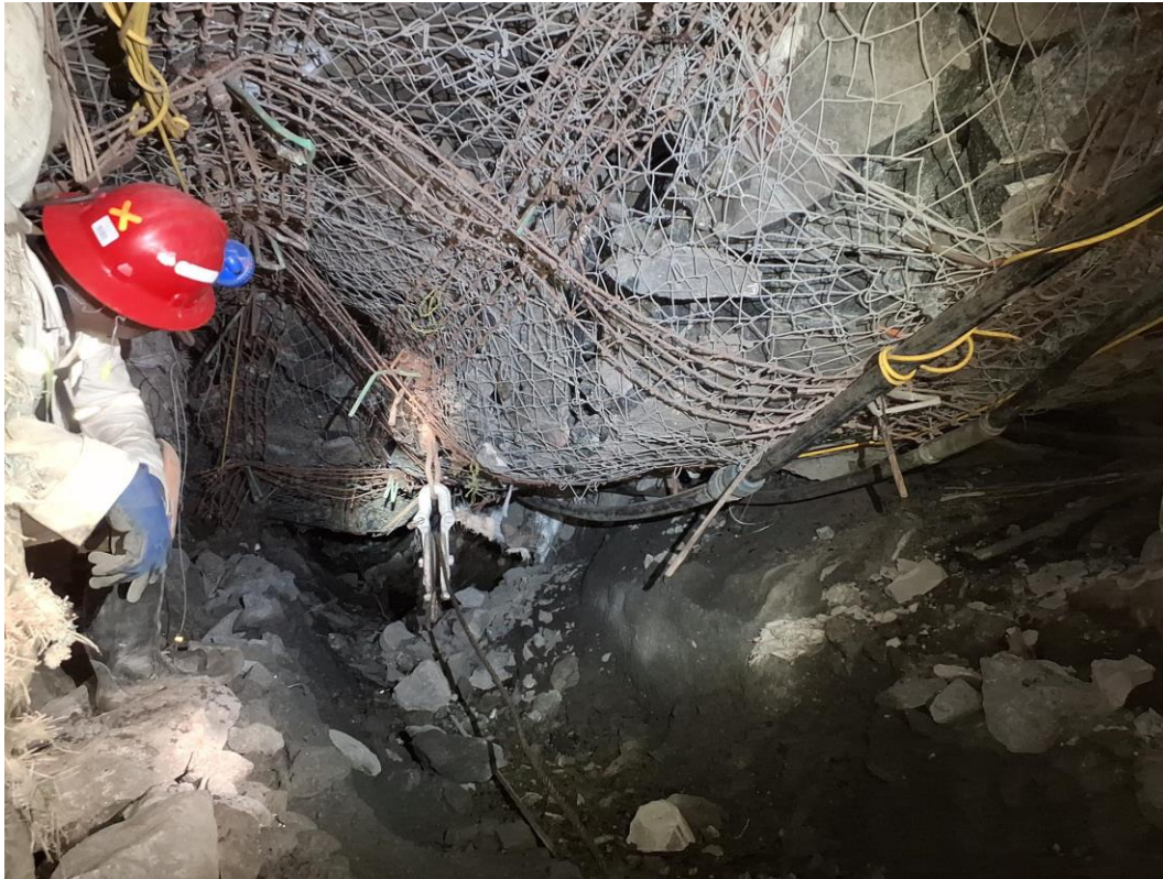
Back Area Collapse
