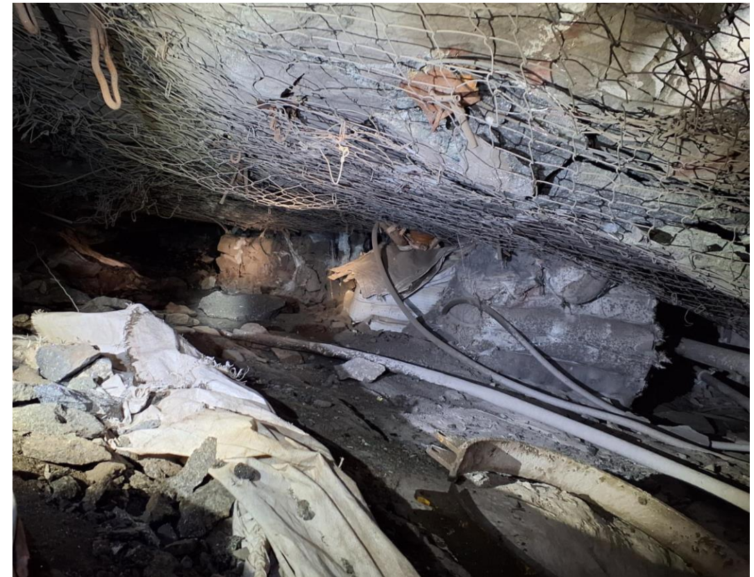
Back Area Collapse
